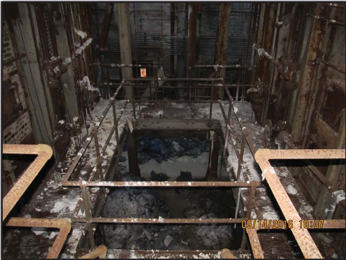
PHOTO 1. English Station - low pressure boiler area.
