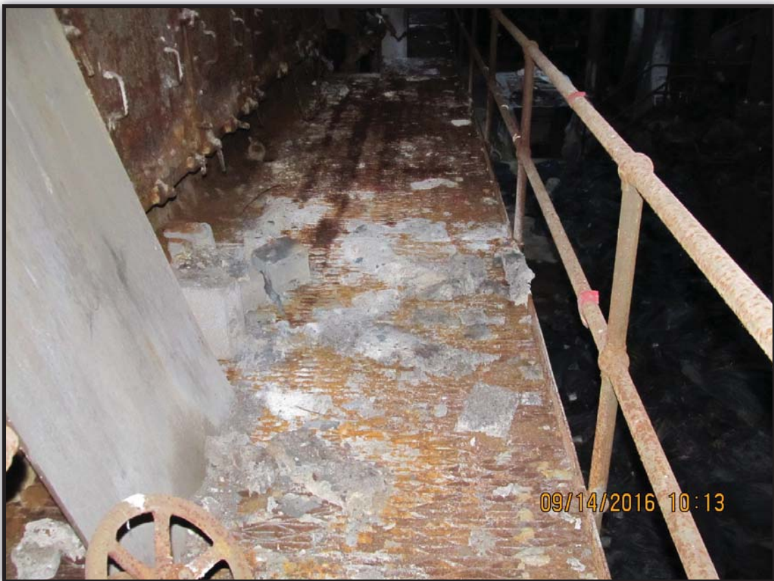
PHOTO 2. English Station - low pressure boiler area.
