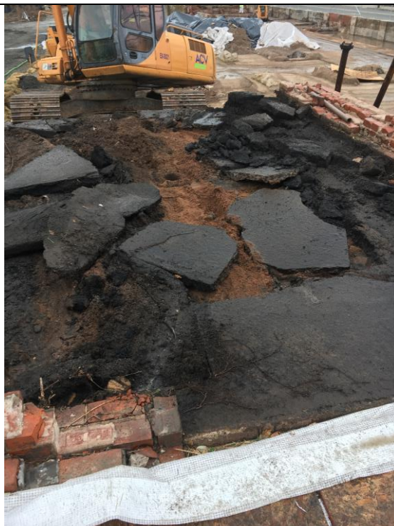
Photo 2: Top of platform with broken asphalt and light brown sand layer prior to sampling.
